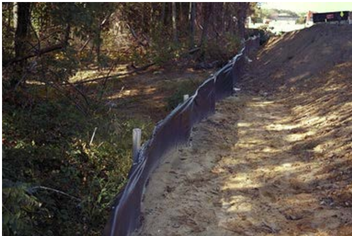
Figure 5.3. Silt fence used as perimeter control to protect wetland (Photo source: MDE, no date)
