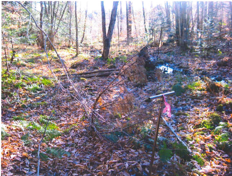
Photograph 2. Two 30-inch HDPE culverts will be embedded 10 inches into the ephemeral stream (located in front of the soil auger) to maintain existing hydrology and habitat connectivity. Photo taken November 18, 2015, looking south.
