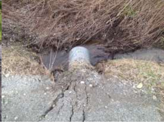
Drainage culvert erosion example
