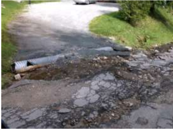
Driveway culvert erosion example
