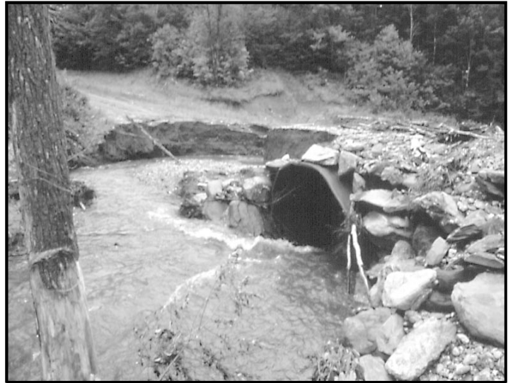
Figure 11. Outflanking Failure at undersized culvert where upstream sediment deposits were observed.
