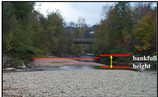
Figure 9. Example of sediment deposit upstream of an undersized bridge that has built to an elevation greater than \frac{1}{2} the bankfull height.
