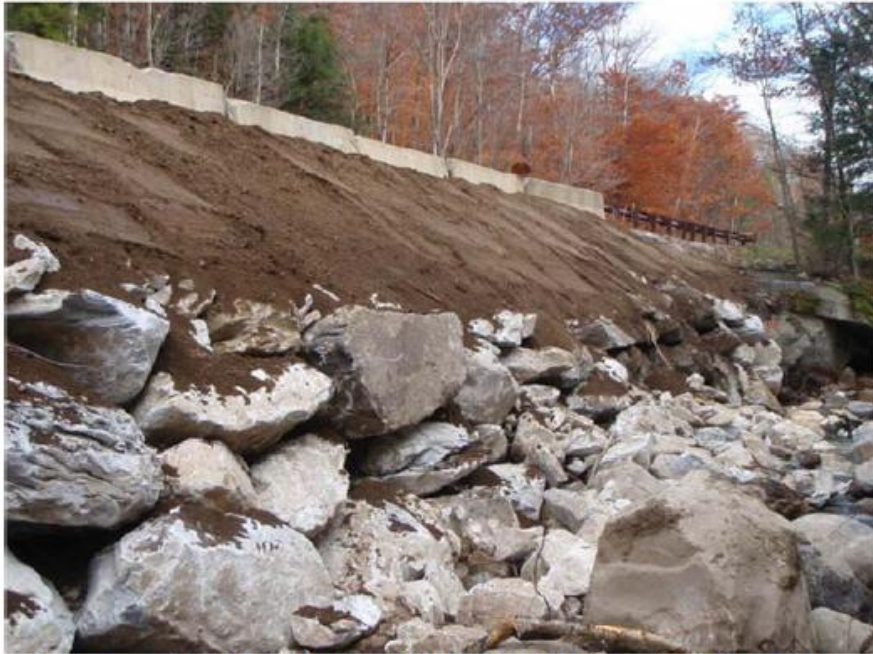
Figure 2. A placed Rip Rap Wall creates lateral channel stability. The steep slope at toe results in less horizontal fill which allows for attainment of full bankfull channel width in confined settings.
