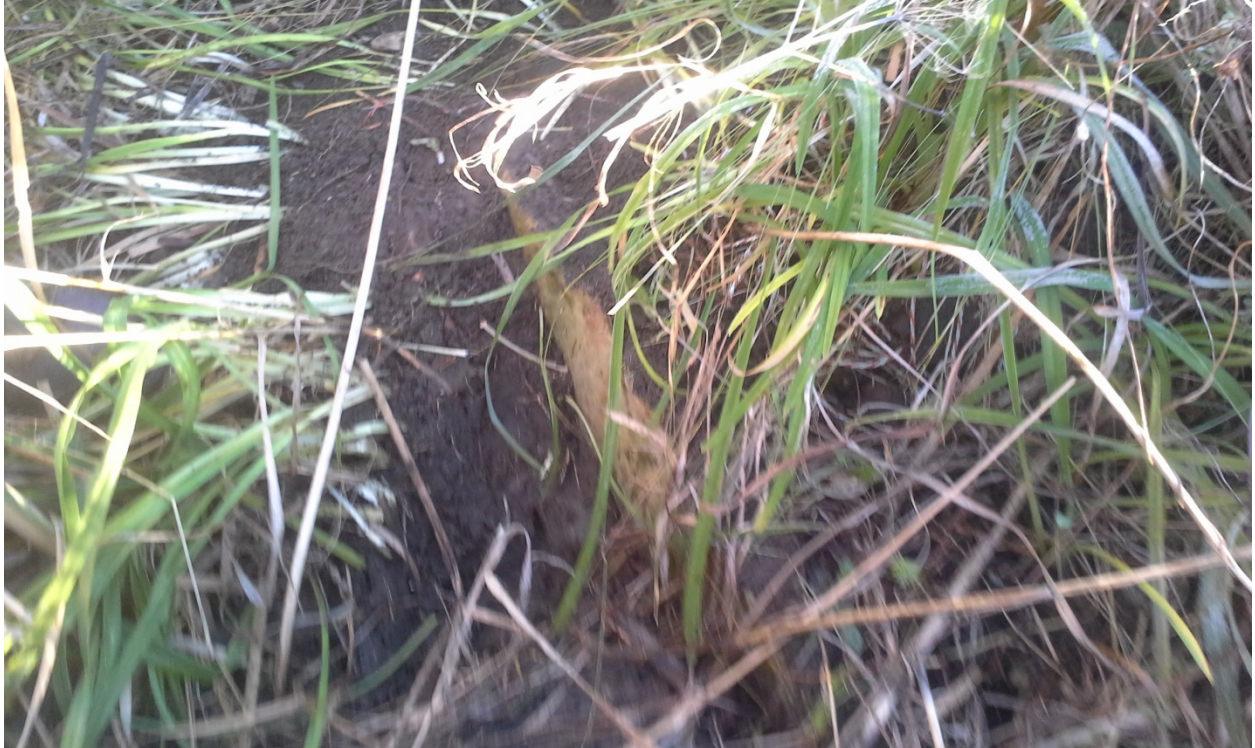
The outlet headwall. The existing culvert is completely silted in and not visible.
