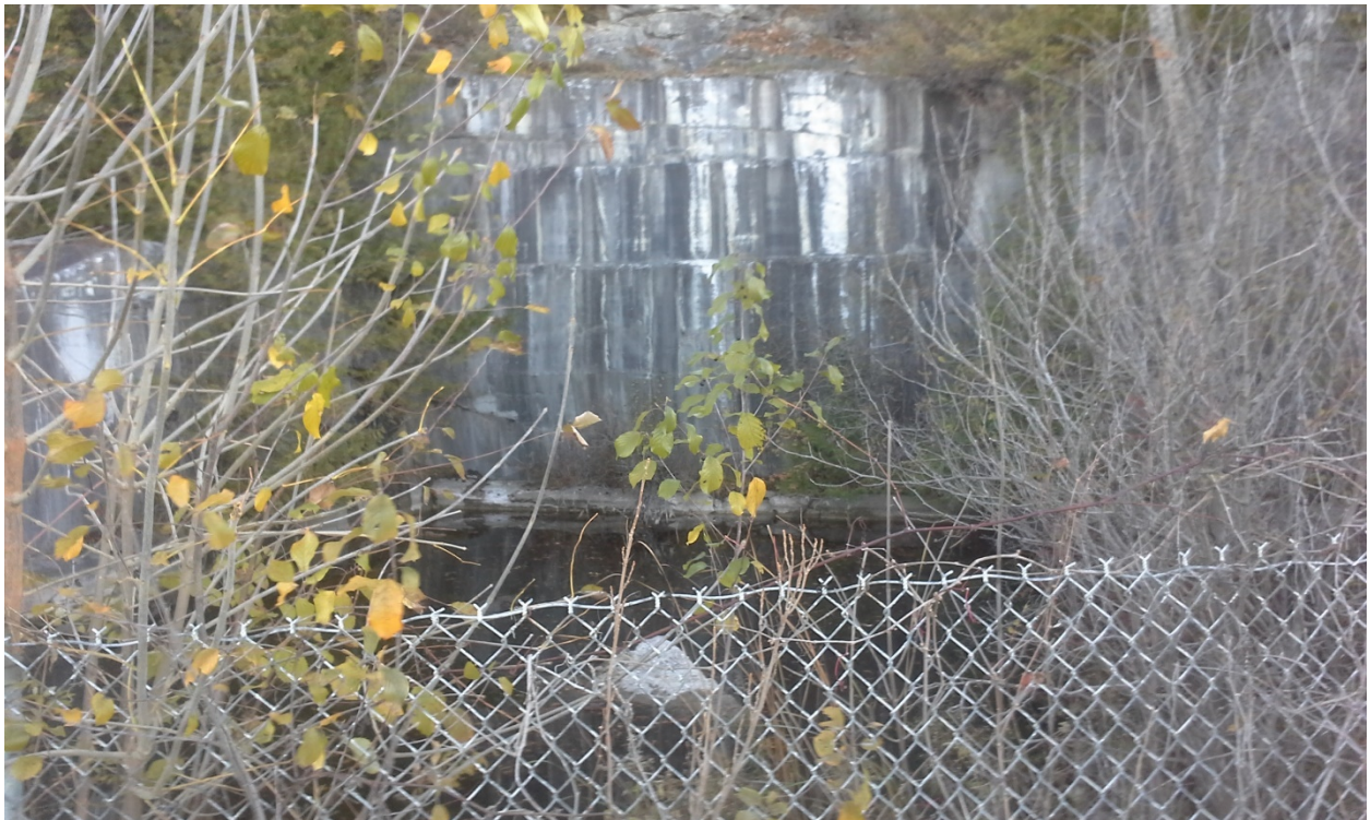
The culvert inlet is not visible. It is located behind the chain-link- fence surrounding the abandoned quarry.
