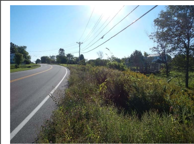
Photograph 1. Existing distribution line along VT Rt 314 at northern edge of the Study Area, looking east
