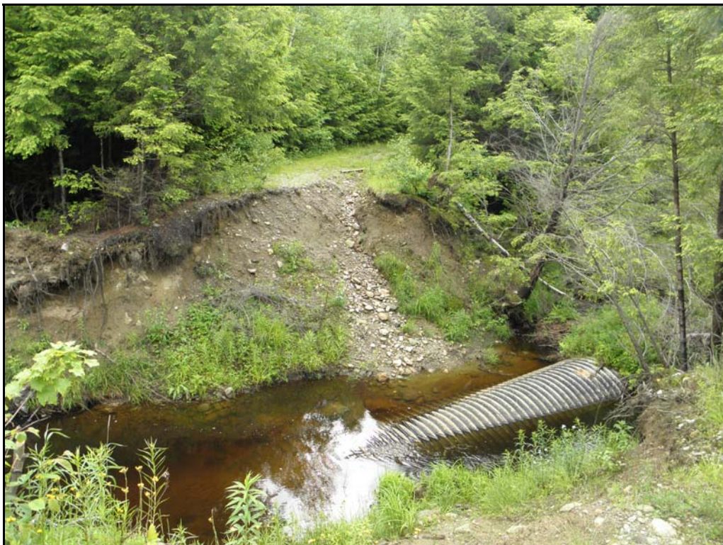
Photo 12. Photo shows the washed out culvert and road that crossed the wetlands at the western end of the East Tract Housing Development. View is to the east.
