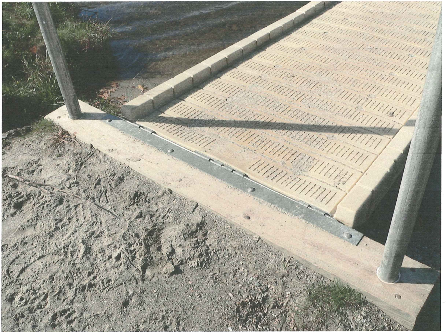
CLOSE UP OF SHORE LAND ANCHOR POINT ON FLOATING SYSTEM
