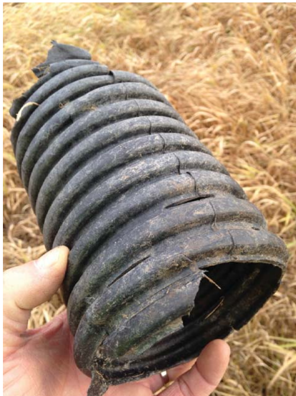
Sub-surface drainage measures and current use diminishes the WL's function and values
