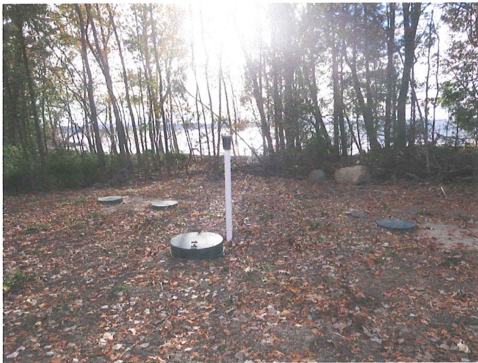
Photo 2: View of Wastewater Collection Tanks at property line view to south.
