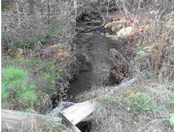
Figure 3 – Beaver Meadow Brook, approaching undersized culvert
