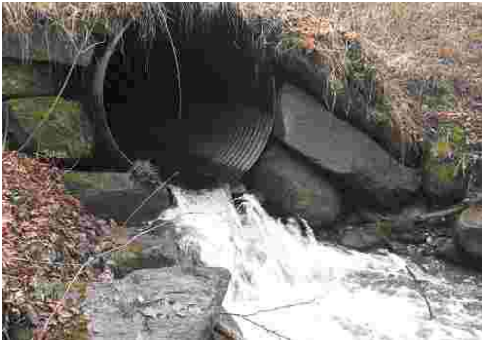
Figure 1– Perched Outlet on Vershire Center Road
