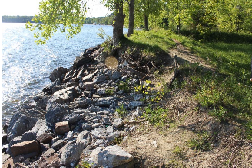
Photograph 4: Representative view of shoreline revetment that will be repaired as part of the Project, location is between jetty and northwest corner of Urban Reserve. View to north. Photo taken 6/1/14 by VHB/Ketterling.
