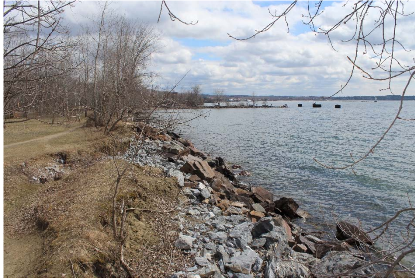
Photograph 3: Representative view of shoreline revetment that will be repaired as part of the Project, location near larger pause place at northwest corner of Urban Reserve. View to south. Photo taken 4/13/13 by VHB/Ketterling.
