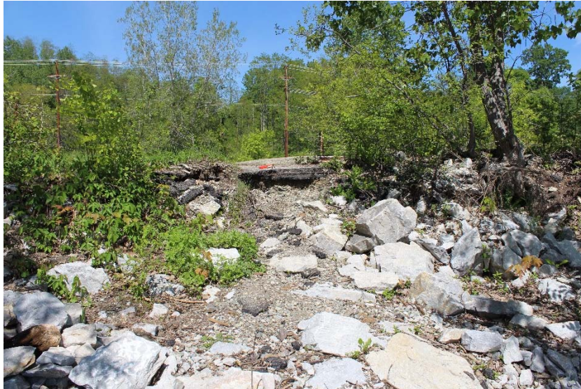
Photograph 5: Representative view of existing shoreline rip rap needing repair and maintenance, approximately at Station 157+50. Photo taken 6/1/14 by VHB/Ketterling.
