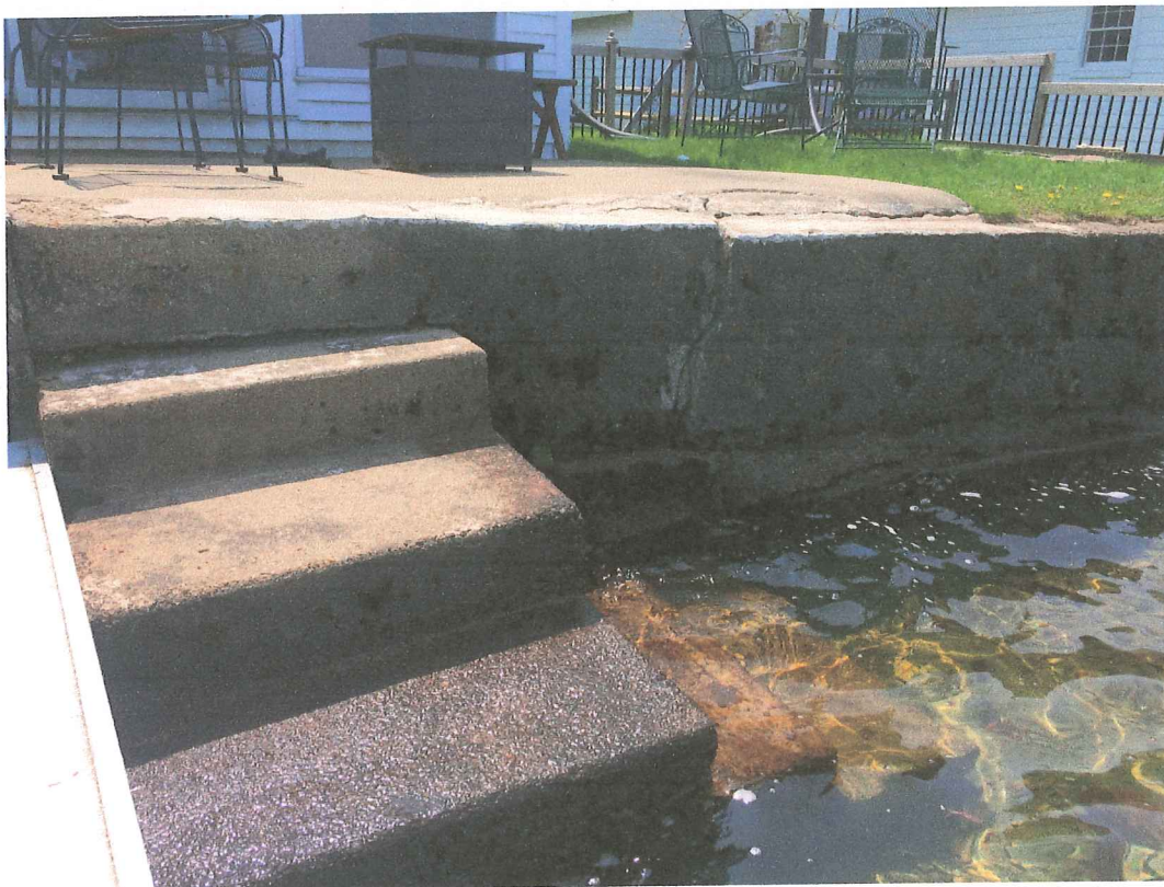
Picture showing stairs that are now leaning and moving
