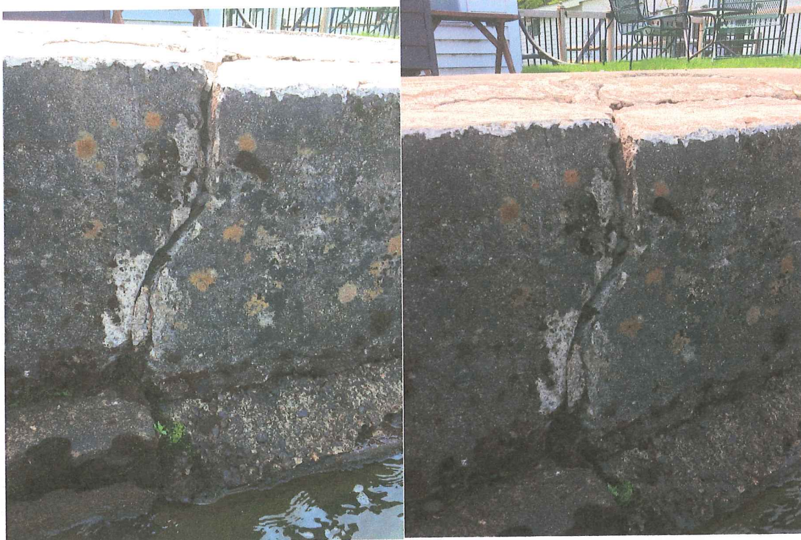
Pictures showing crack in wall that is growing annually
