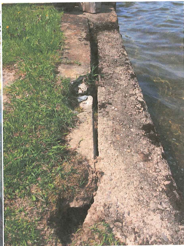
Picture of west showing separation and cracking
