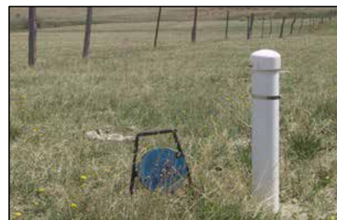
A monitoring well at the ground surface.
