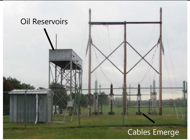
Photograph 2. Looking west at existing Terminal Station. Existing submarine cables emerge below wooden structure, and the oil reservoirs are located on the metal structure to the left.
