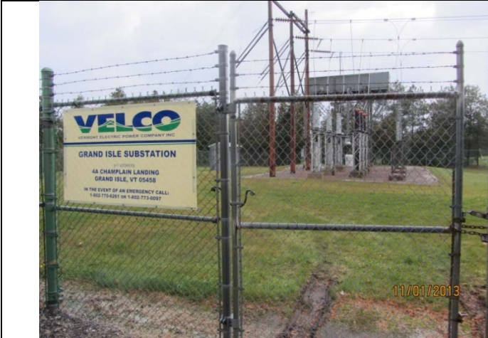
Photograph 1. Looking north at the VELCO Grand Isle Terminal Station.
