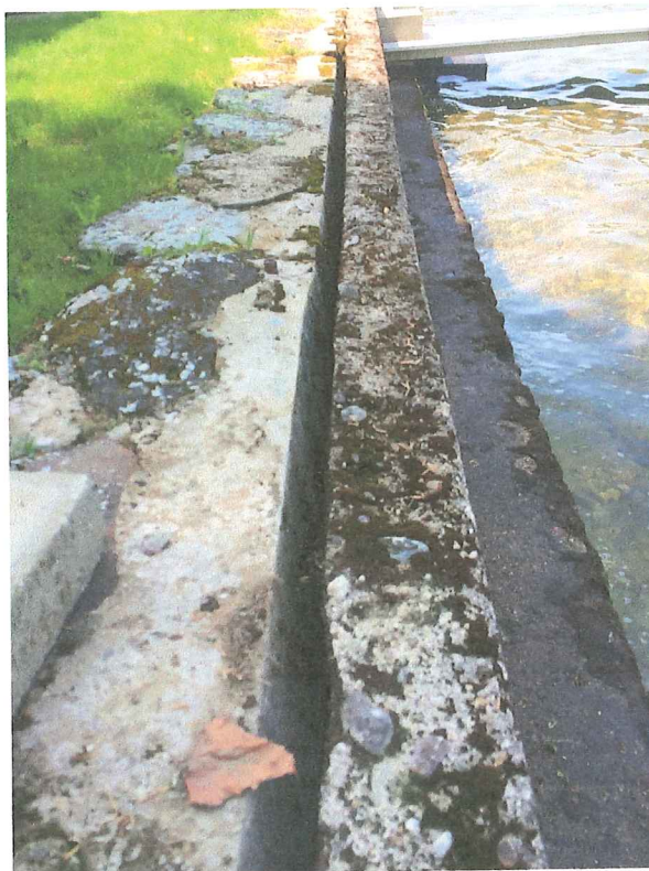
Picture of east end showing wall separation
