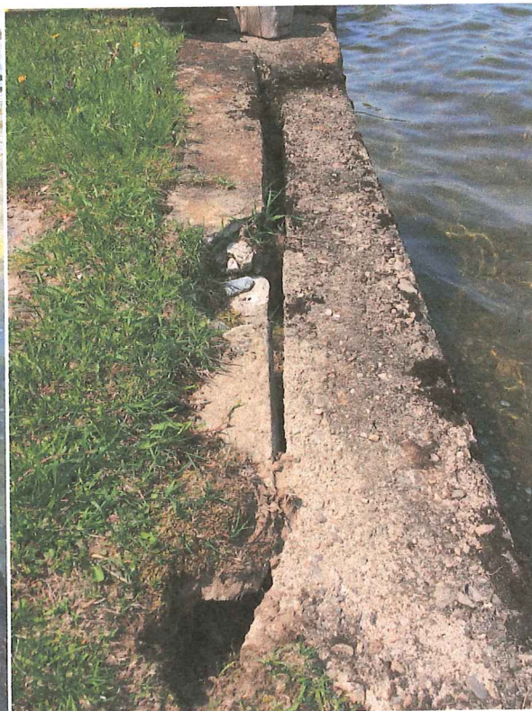
Picture of west showing separation and cracking
