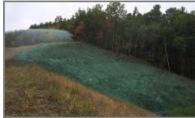
Installation date, Sept. 21st
