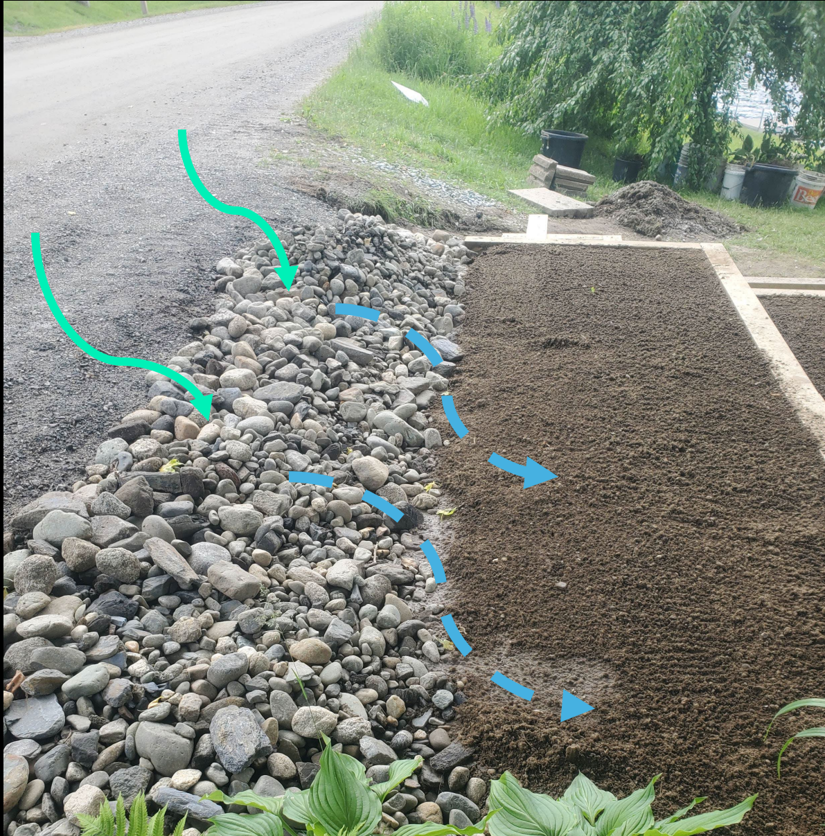
...enters the beds via a stone inlet & infiltration trench.
