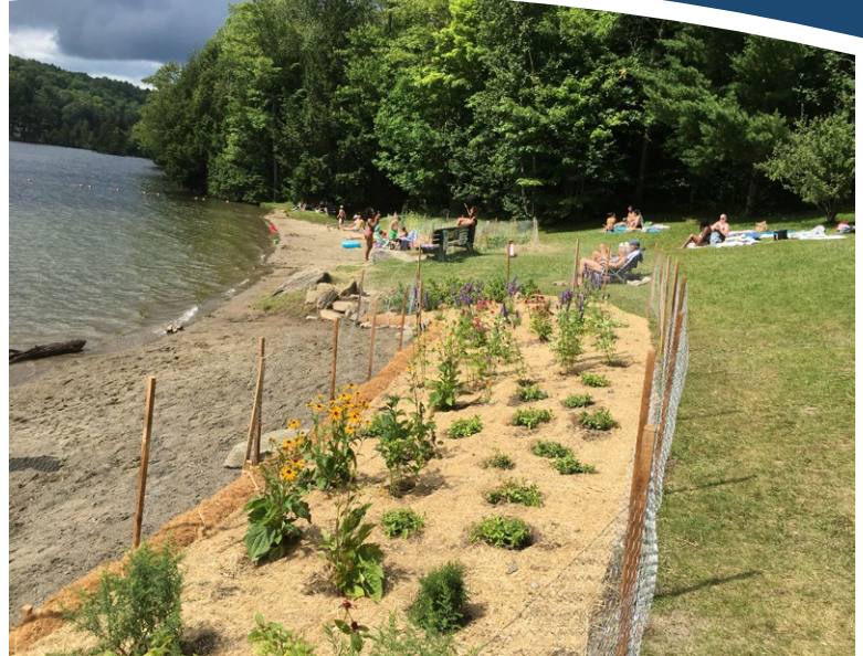
INSTALLATION. Stabilized with fiber coir rolls, erosion control blankets, native plantings, and stone step access.
