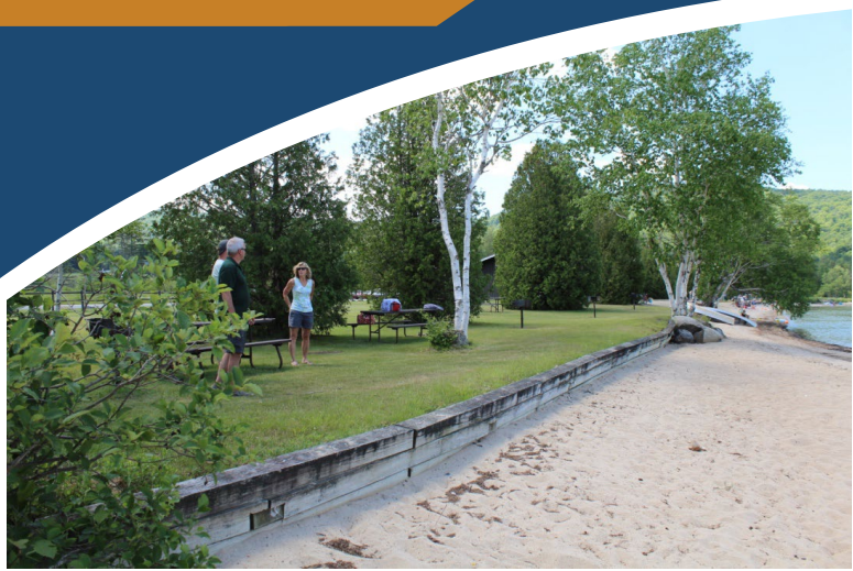
Failing retaining wall at Brighton State Park, Island Pond.
