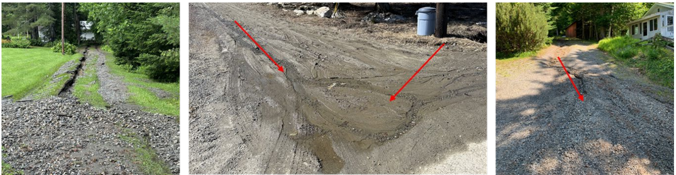
Figure 23. Several unpaved driveways in the watershed are graded so that water runs down the center of the driveway rather than shedding water off of the driveways to green areas, resulting in erosion and sediment transport especially during larger storm events. Red arrows show the direction of flow.
