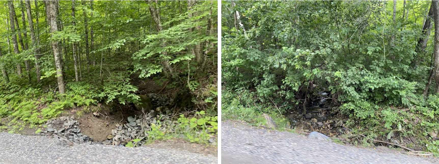
Figure 29. Unstable stream banks and direct connections between roadside ditches and streams are recurring problems in the watershed.
