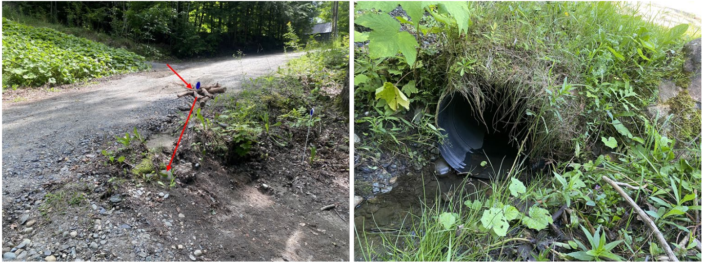
Figure 21. Absent (left; see flow paths across road highlighted with red arrows) and undersized (right) culverts have resulted in erosion during larger storm events.
