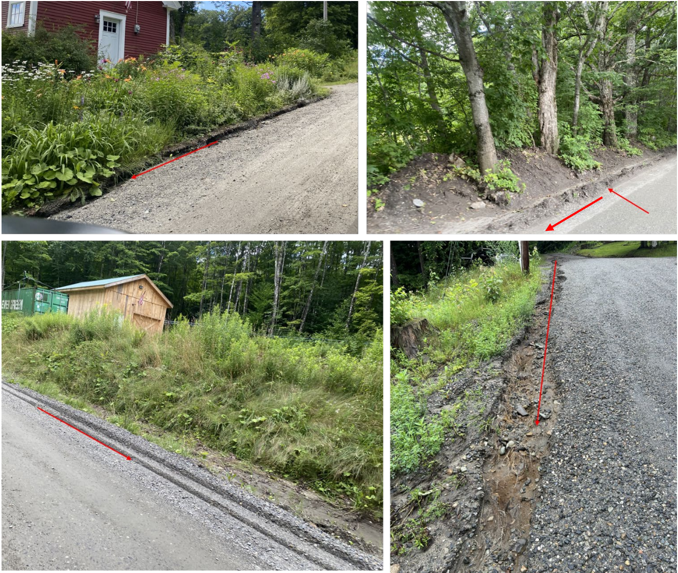
Figure 24. Improper grading and the creation of grader berms that restrict flow to the road result in erosion and sediment transport. Red arrows show the direction of flow.
