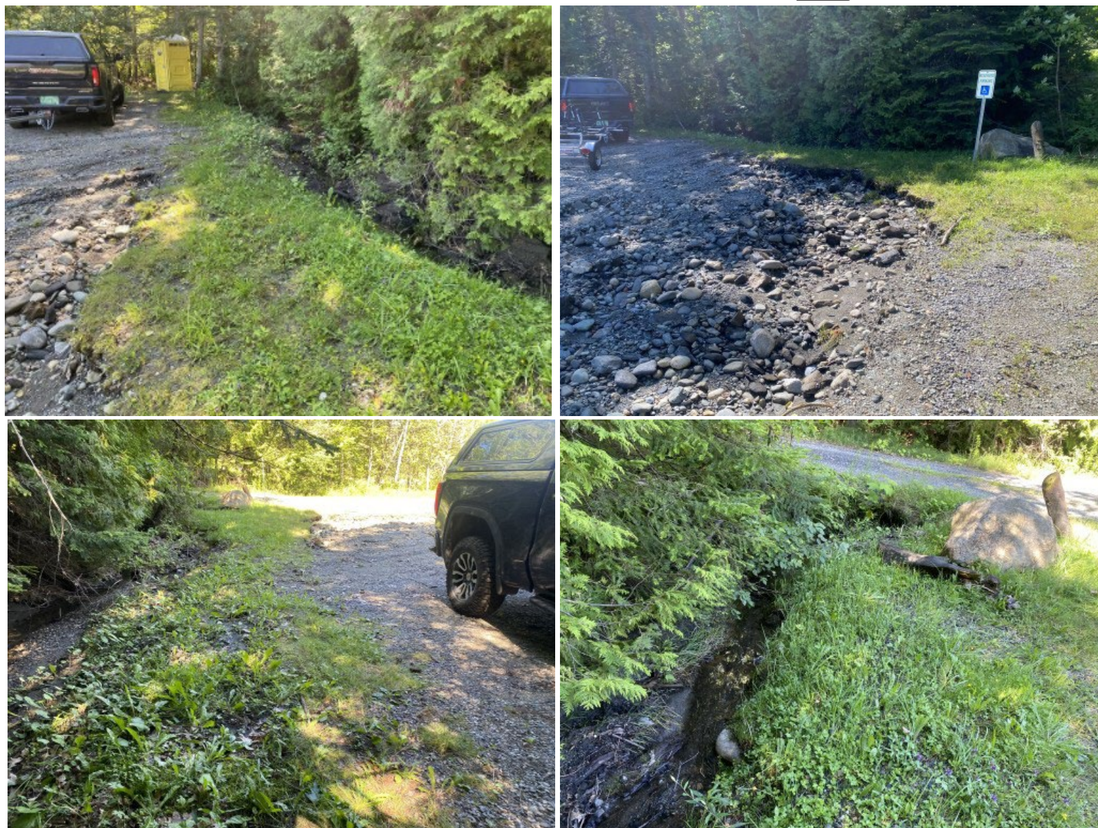
Figure 30. The Fish and Wildlife Access parking area abuts a tributary that has been artificially straightened and lacks a robust riparian buffer (upper left and lower left) and has an undersized culvert (bottom right) that contributed to the stream jumping its banks during the July 2023 storm, which caused significant damage and sediment transport (top right).
