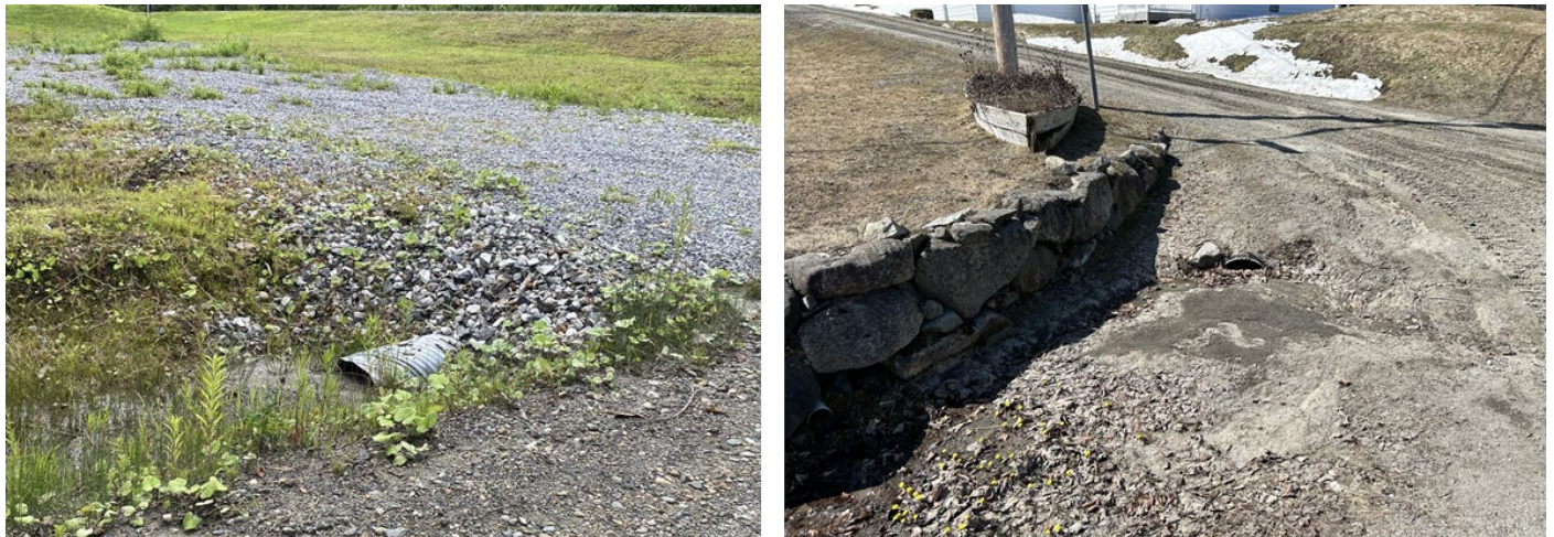
Figure 22. Clogged culverts cannot transport stormwater effectively and can lead to scour and flooding damage in adjacent areas and the transport of sediment to Shadow Lake.
