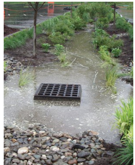
PARKING MEDIAN BIORETENTION CELL MONTPELIER, VERMONT
