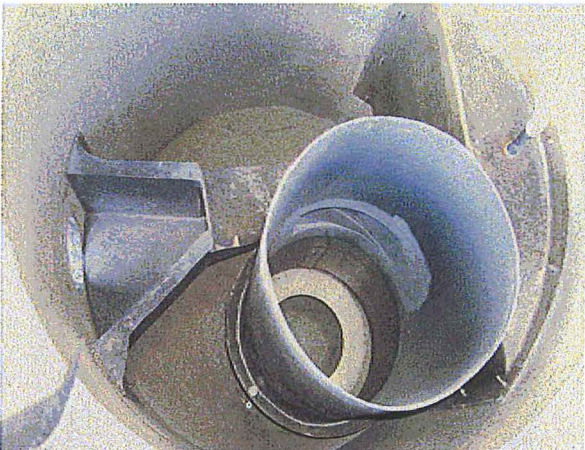
STORMWATER TREATMENT STRUCTURE
