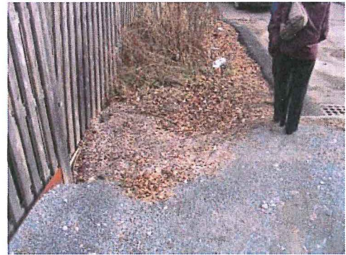
Break-away fence at end of Harrington Terrace: Build-up of leaves and sediment pushing up against fence, damaging hinges
