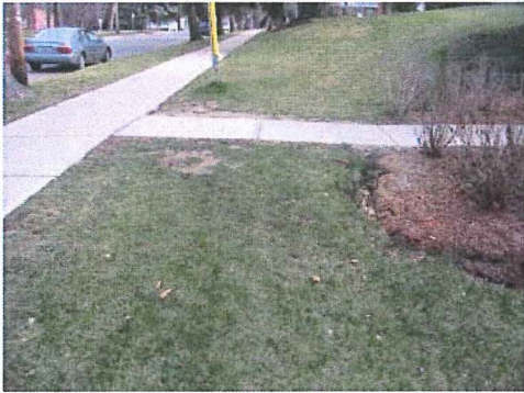
Entrance walk to S.D. Ireland Center, Maple Street side -Ties-in high point in city sidewalk causing storm water to flow toward building
