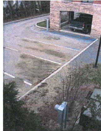
Behind Main Street Suites: Paved walkway showing evidence of erosion
