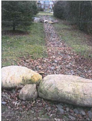
Stone drainage swale w/ boulder check dams
