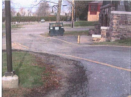
Driveway behind Hill Hall: Undulations in pavement, artificial low point corner of building
