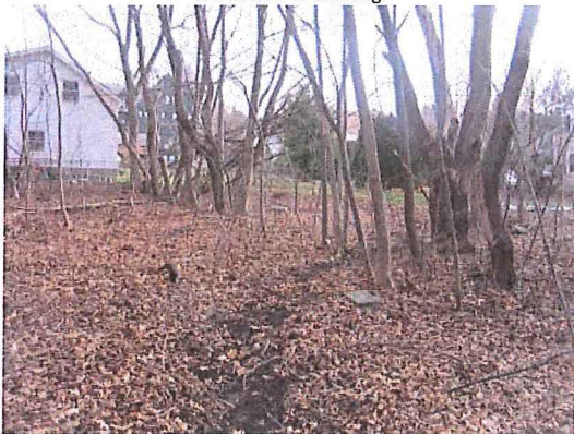
Rowell Annex: Off-site erosion as a result of channeled runoff, from south side of building
