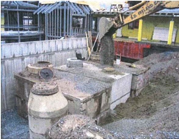
STORMWATER RETENTION TANKS
