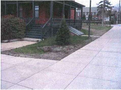
Ground area around/behind Aiken Hall -sediment build-up around CB, more foot traffic erosion
