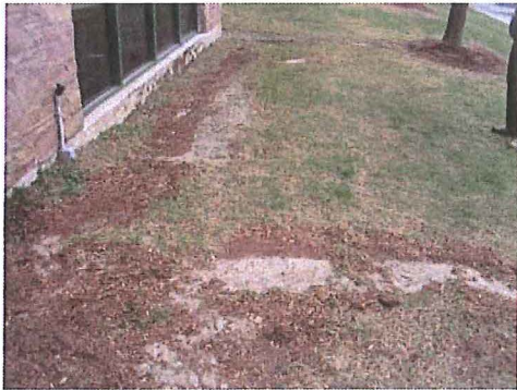
Ground area around Hauke Family Campus Center: Rooftop runoff causing erosion of ground area and sediment build-up
