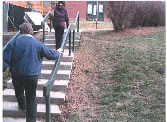
Stairs behind Freeman Hall Slope erosion due to foot traffic, uncollected storm water runoff
