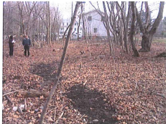
Rowell Annex: Off-site erosion as a result of channeled runoff, combined from north, south
