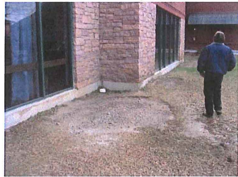
Ground area around Hauke Family Campus Center: Rooftop runoff causing erosion of ground area and sediment build-up
