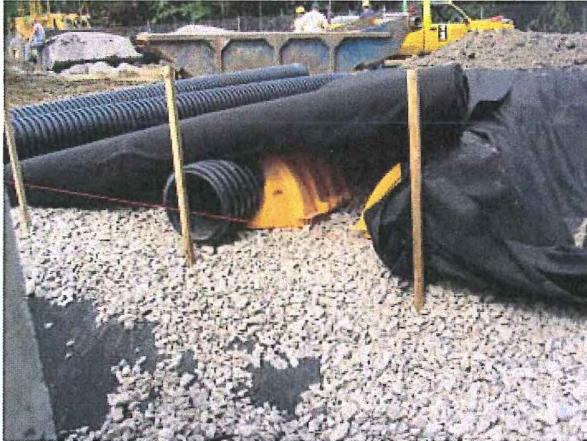
STORM WATER INFILTRATORS
