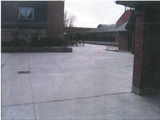
Terrace behind Bader Hall: Large impervious area w/ no disconnection of runoff
