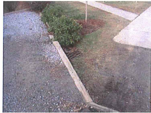
Catch basin near Carriage House, behind Joyce/Freeman CB in non-functional location
