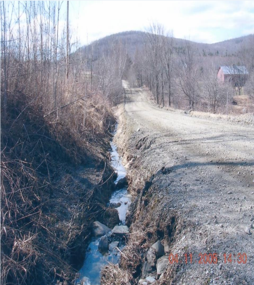
Eroding roadside ditch
