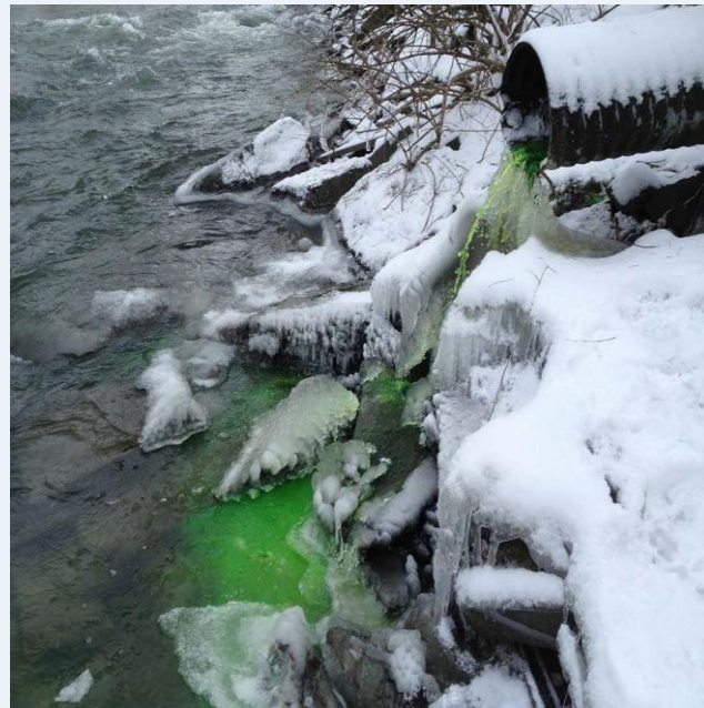
Illegal discharge of untreated sewage, dyed green for the assessment
