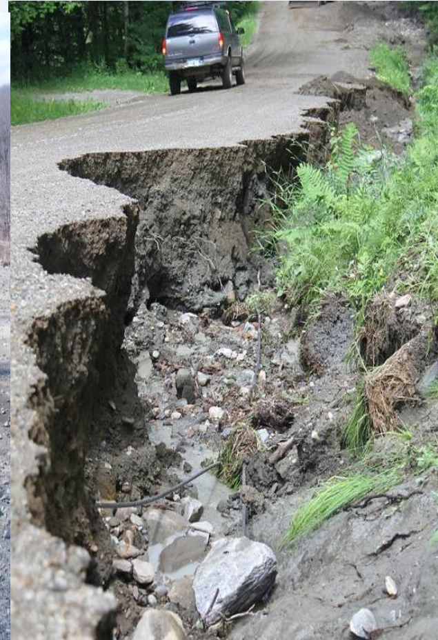
Storm-damaged gravel road
