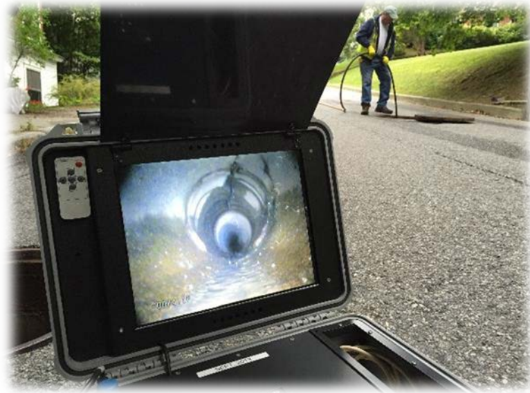
Town of Bennington Water Dept. crew uses a camera to identify a leak in the line near SMH-1450. Cracks in the pipe are visible in the photo.
