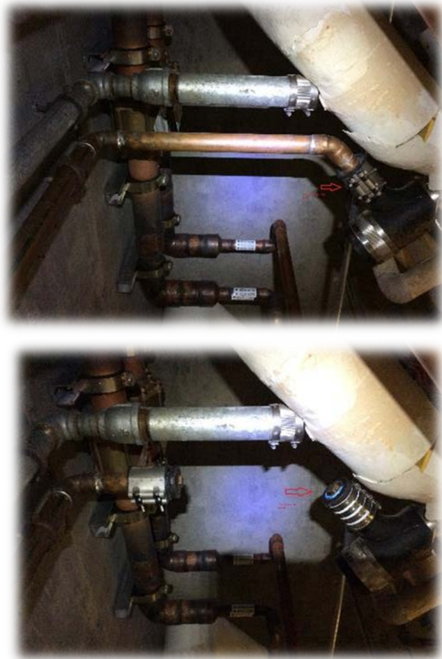
Before (top) and after (bottom) photo of the improperly connected sink at the hospital.
