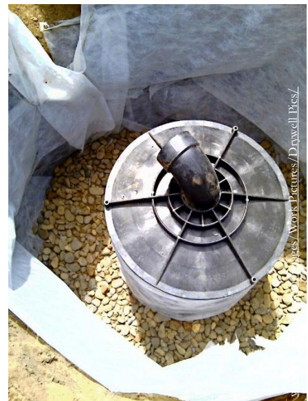
Installation of a drywell, including a manufactured tank, gravel jacket, and filter fabric.
