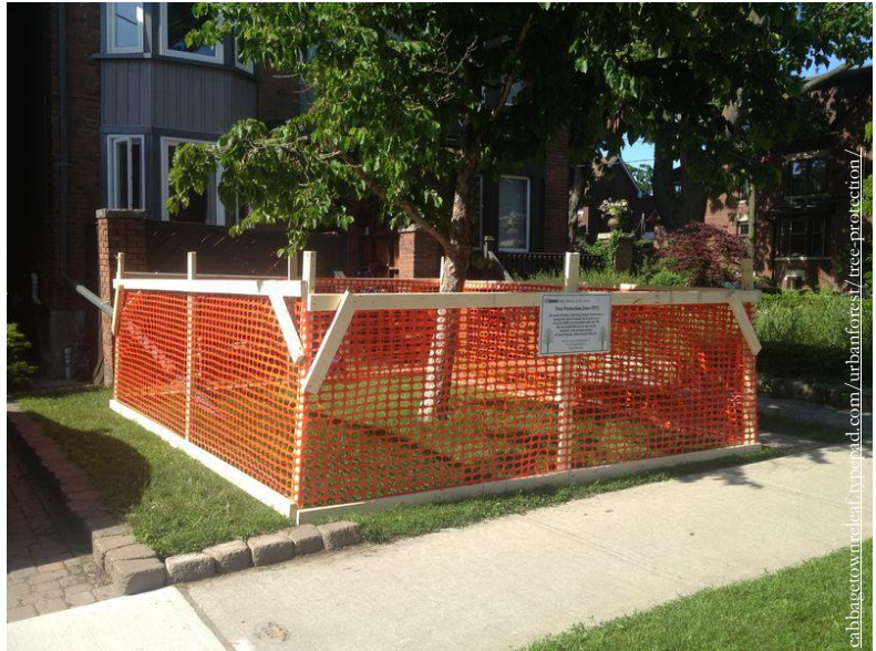
Protecting trees to be retained from damage and disturbance during construction activities is critically important for the trees' long-term health and performance.
