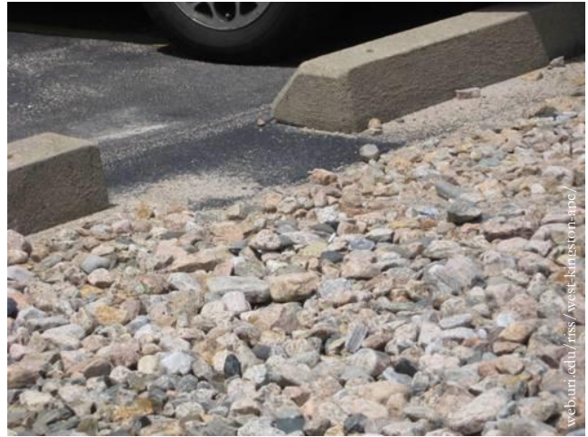
A gravel diaphragm catches runoff and distributes it as sheet flow to the filter strip, settling out sediment and preventing erosion.
