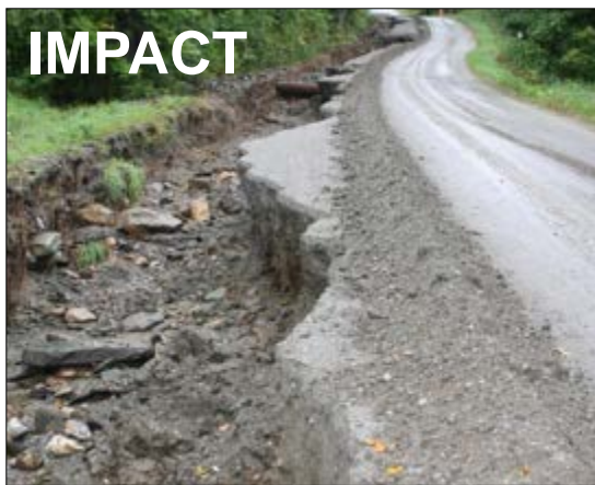
Eroding roadside ditch
