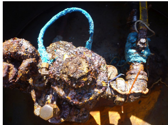
Acetic Acid Corrosion
