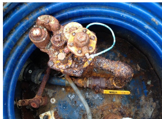
More corrosion from acetic acid
