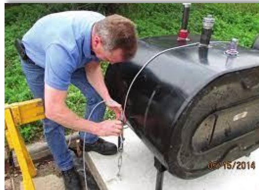
Above: An installer performing a wire rope tie-down which is another way to secure a tank in a flood-prone area
