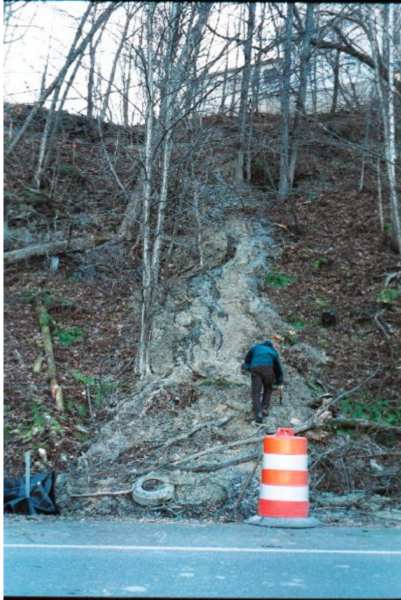
Figure 3. Earth flow originating in central part of slide and flowing down to culvert on east side of State Route 15. November 10, 2003.
