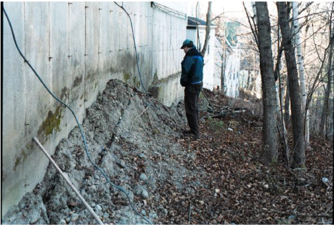
Figure 7. Fractures in earth at lower side of foundation of Wiggins house. November 10, 2003.
