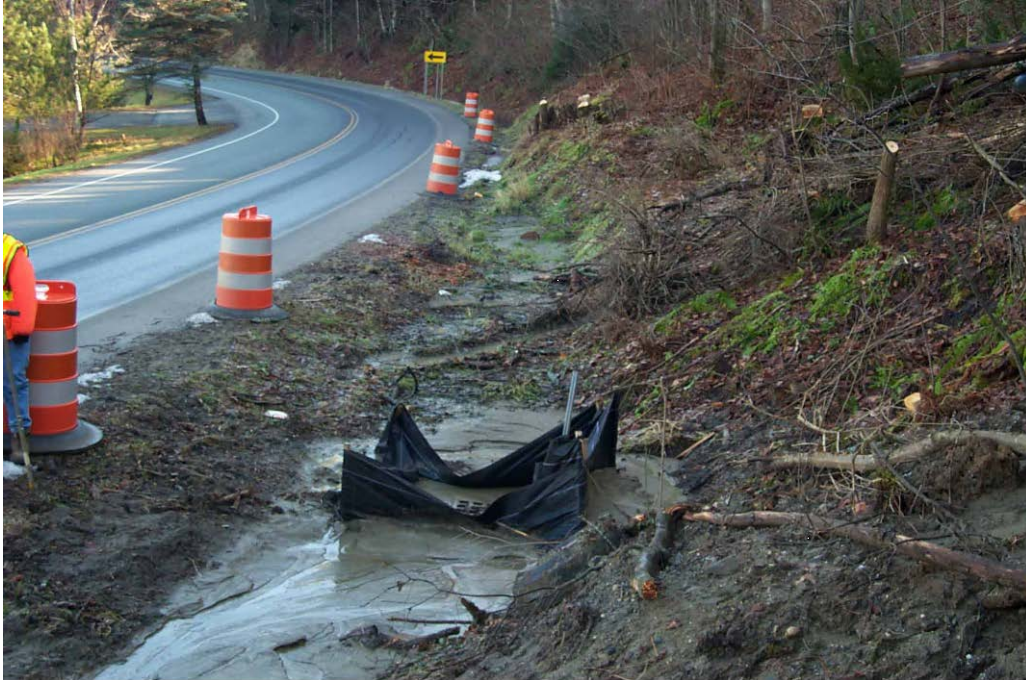
Figure 4. View of sediment from slide washing into catch basin on south side of Route 15. Looking east. November 21, 2003. Photo by Vtrans.
