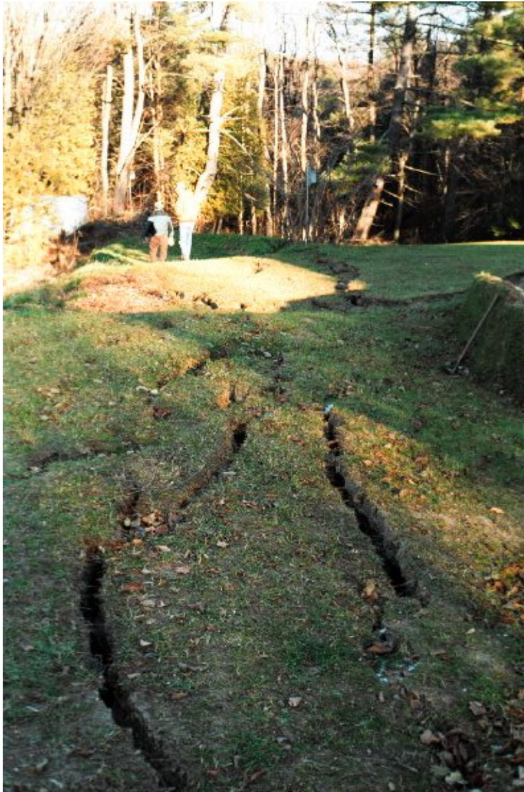
Figure 10. Fractures in artificial fill on northwest side of Holmes residence. Photo looking east-northeast. November 10, 2003.
