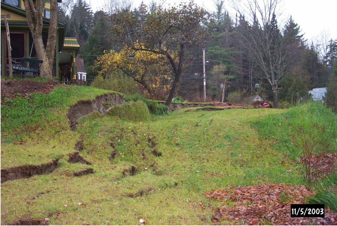
Figure 11. Uppermost scarp at Holmes residence. View looking southwest. November 5, 2003. Photo by VAOT.
