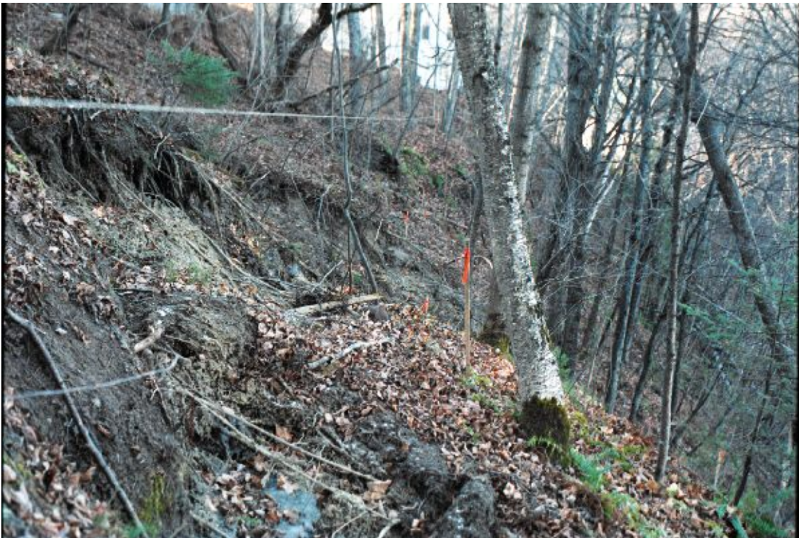
Figure 5. Recent scarp formed within landslide. Photo looking northwest. VAOT reference strings are shown on left and right sides of photo. Stakes were originally under the strings and have moved downslope since they were installed. November 10, 2003.
