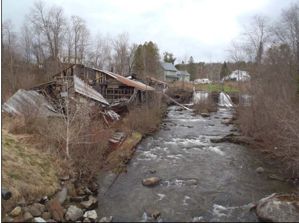
Figure 7. Looking upstream at an abandoned sawmill with a dam built on ledge. Site is on Winooski River north of Sawmill road, downstream of Lower Cabot.
