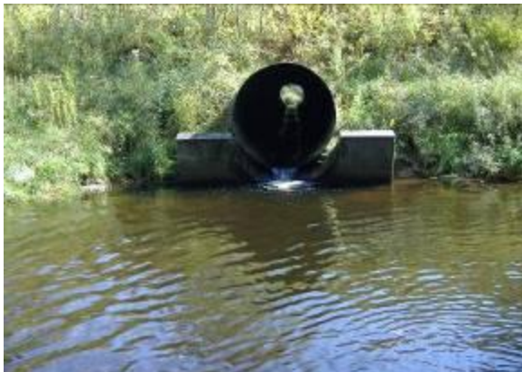
Scour Pool, State Park Road
