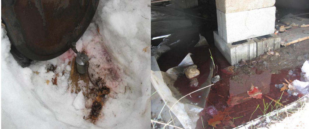
200 gallon kerosene leak at mobile home. Kerosene migrated under home. Athens, April 2008
