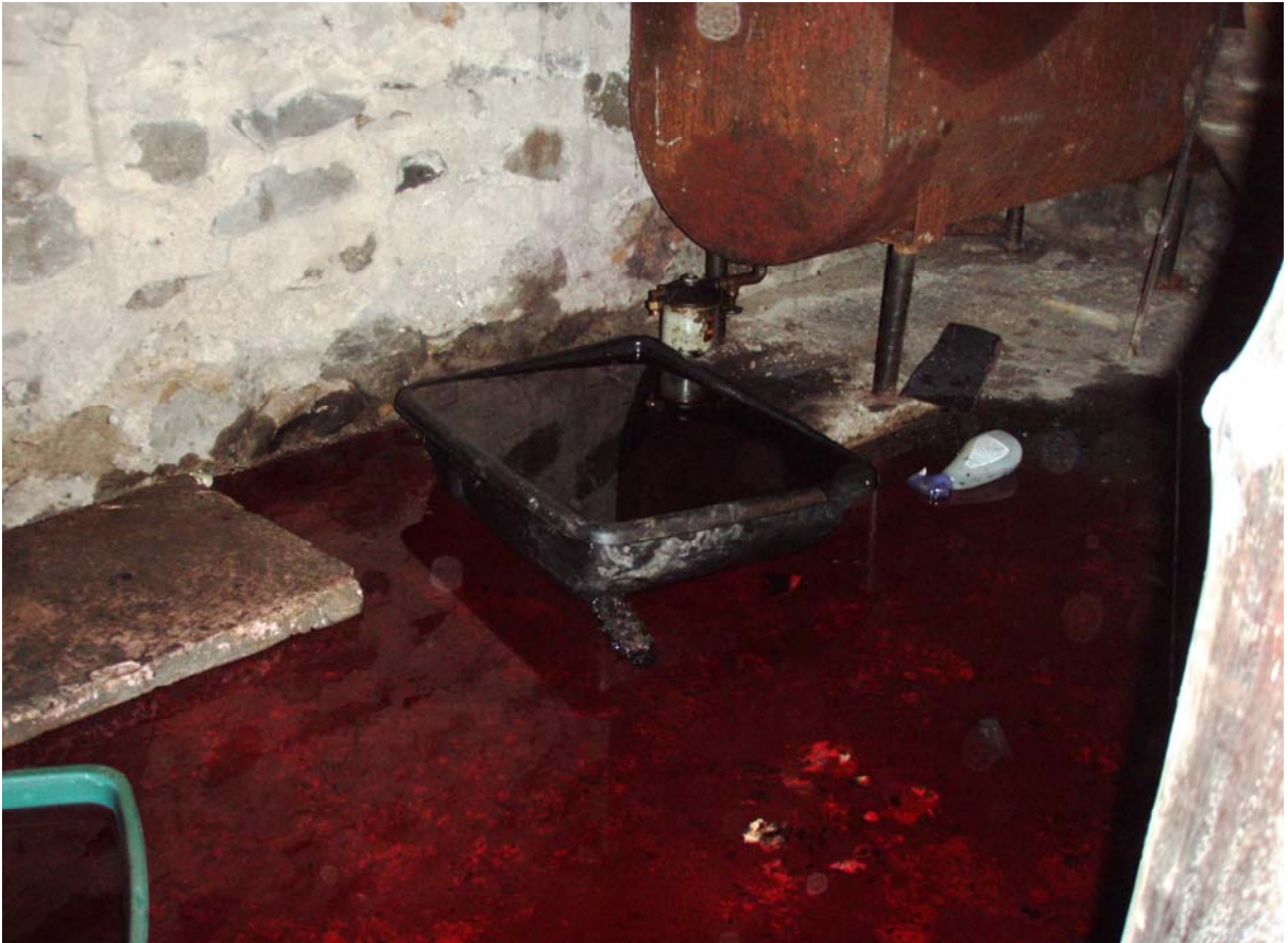
220 gallon heating oil release from residential tank in St. Albans, October, 2008
