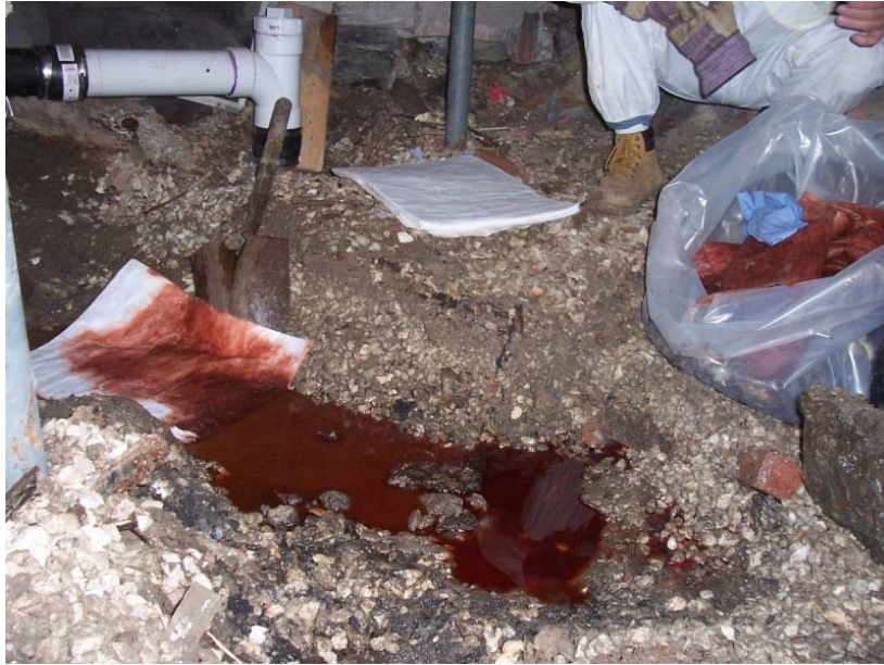
50 gallon heating oil spill in the basement of home in Vergennes, December, 2008
