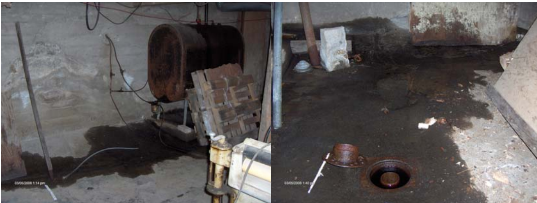
175 gallon fuel oil release. Product migrated outside home via floor drain. Barnet, March 2008
