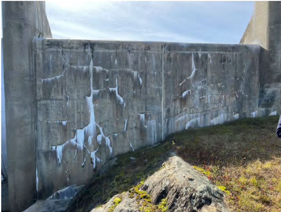
Fig. 4-3. Cracks on Upstream Side of Monolith M1 and M2
