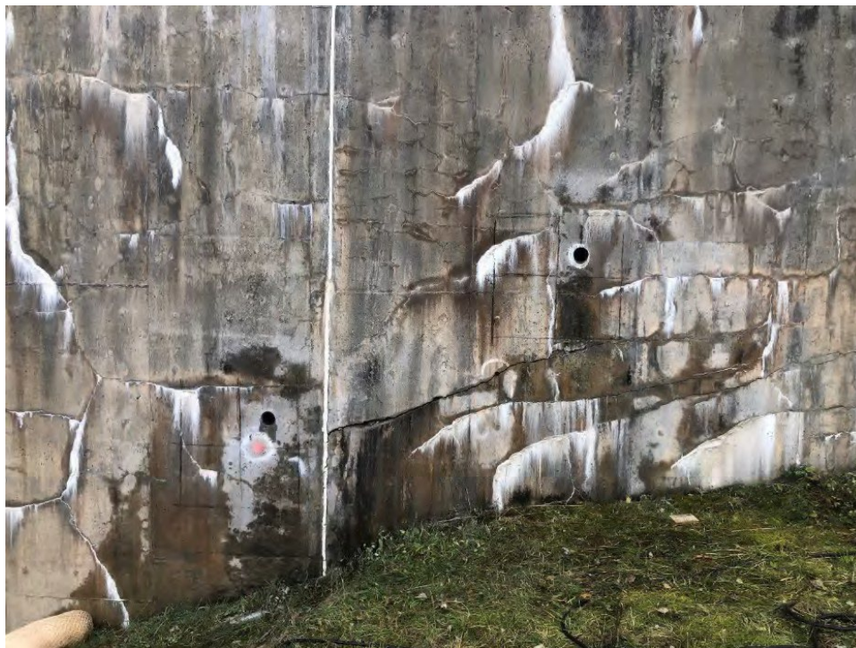
Fig. 4-4. Close-up of cracks on Upstream Side of Monolith M1 and M2
