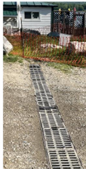
Concrete and steel trench drain
