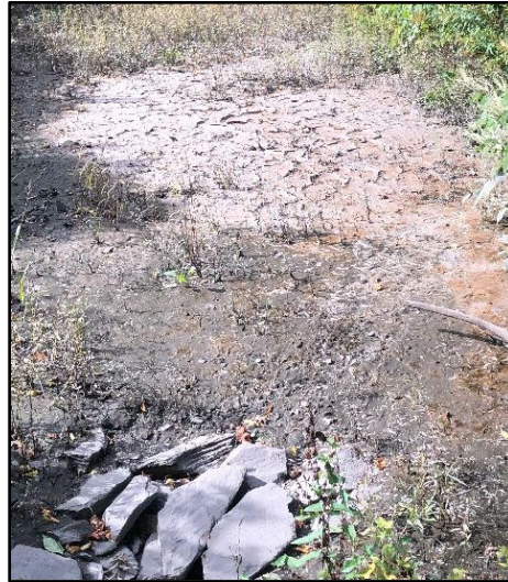
Example photo of bioretention with Severe sediment accumulation and clogged filter media/natural soils.
