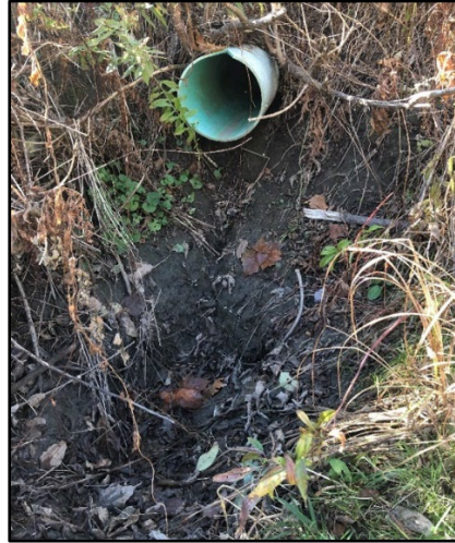
Example photo of Minor erosion at the outlet.
