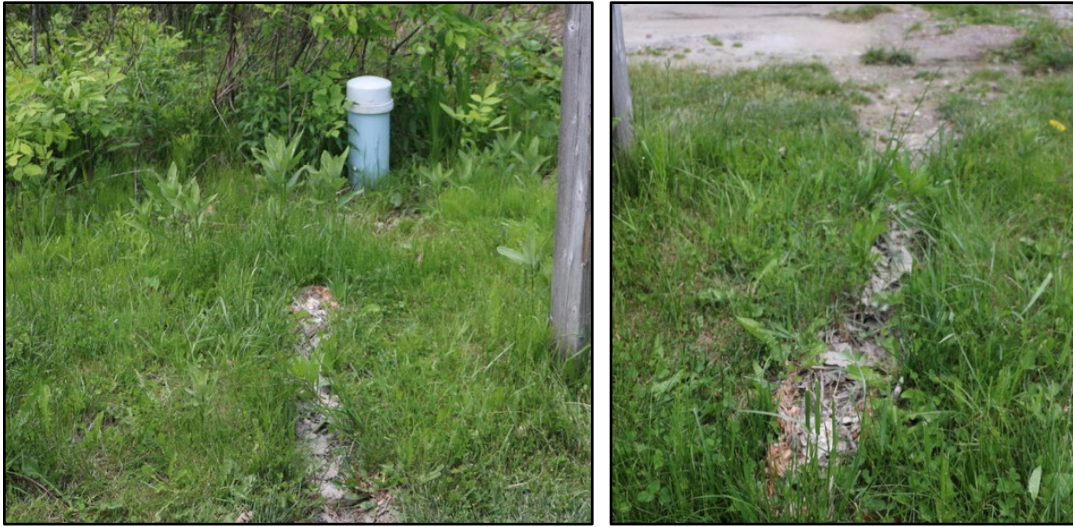
Example photos of Rill 1 erosion. [Left] looking in towards bioretention. [Right] looking out towards impervious surface.
