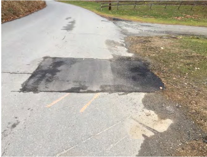
Figure 3. Pavement patch on Fern Street over apartment building's new sewer service connection
