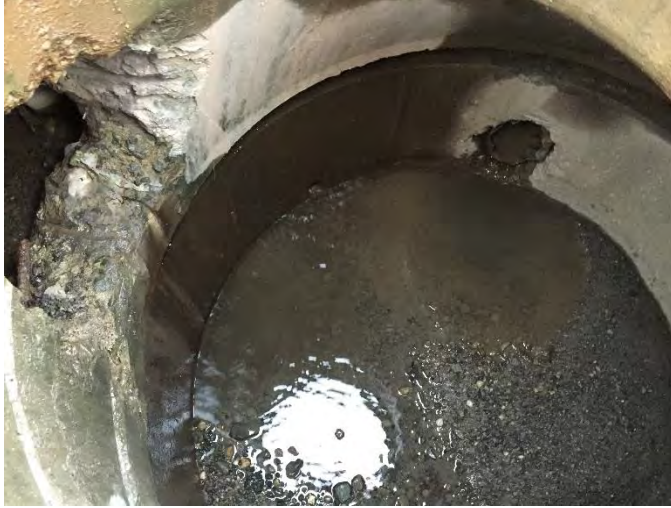
Figure 4. Deteriorated pipe penetrations in catchbasin CB1
