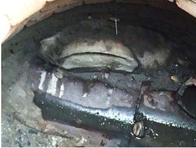
Figure 2. Manhole MH1—a gap in the plug is visible in the pipe in the 11:00 position
