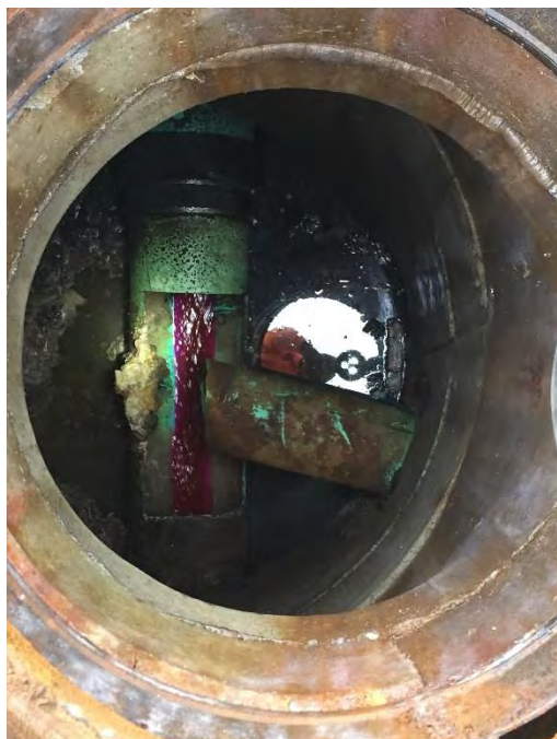
Figure 1. Sanitary manhole showing dye from service station pit drain
