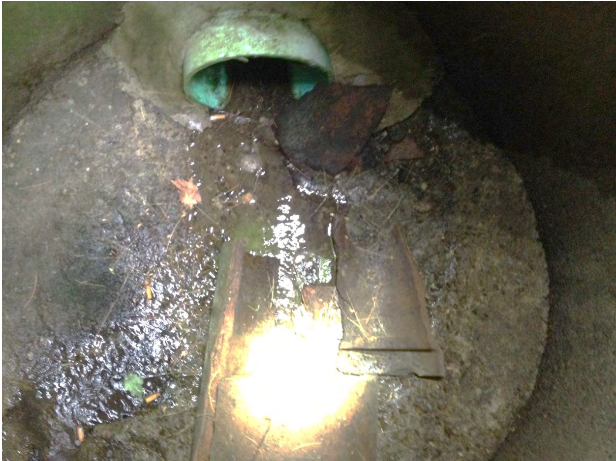
Stormwater manhole at the Newport Elementary School with visible wastewater solids, June 16, 2015
