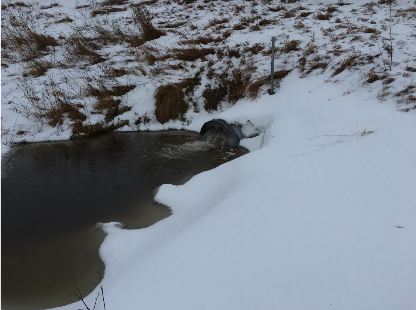
IMG_1732, Taken on 1-23-2018 by John D. E. Roberts . View of the 30” culvert under Route 236 that is frozen, except for two small holes
