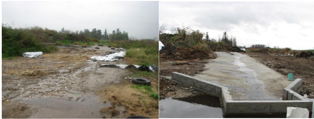
Figure 1. BMP for silage leachate collection system, before and after.
