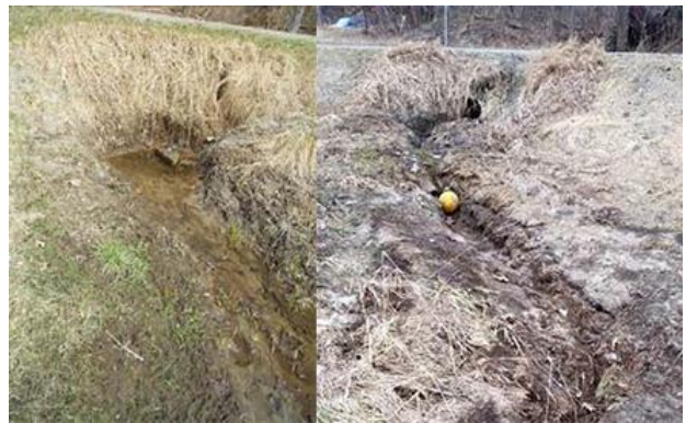
Figure 27. Before (top) and after (bottom) installation of bioretention system on Morey Road in Hyde Park, completed by Lamoille County Conservation District
