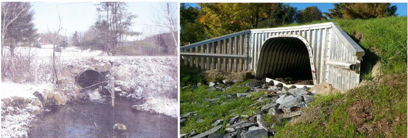
Figure 29. Before (left) and after (right) replacement of stream culvert at Junction Hill Road in Cambridge, completed by the Town of Cambridge
