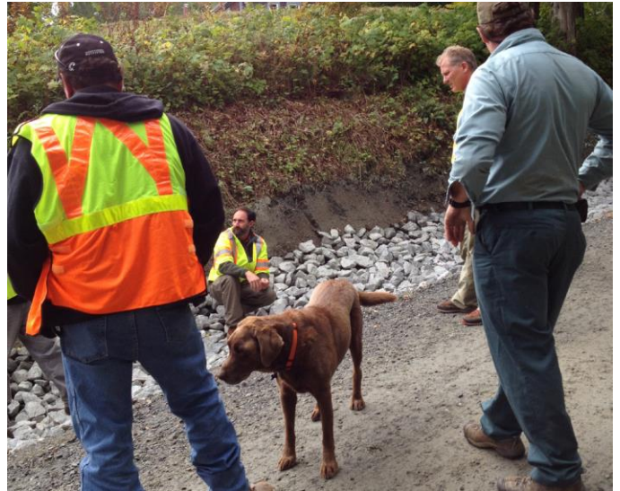
VTrans and DEC staff visiting a stone-lined ditch during a site visit
